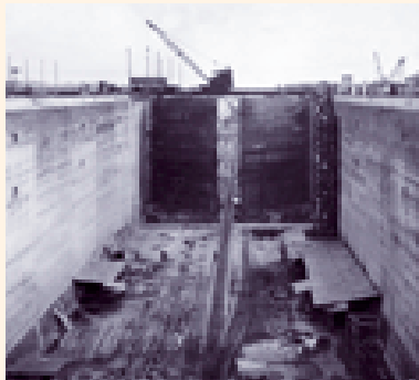
The locks, whose steel gates rise six stories high, can hold as much as 26 million gallons of water—enough to supply a major U.S. city for one day.
